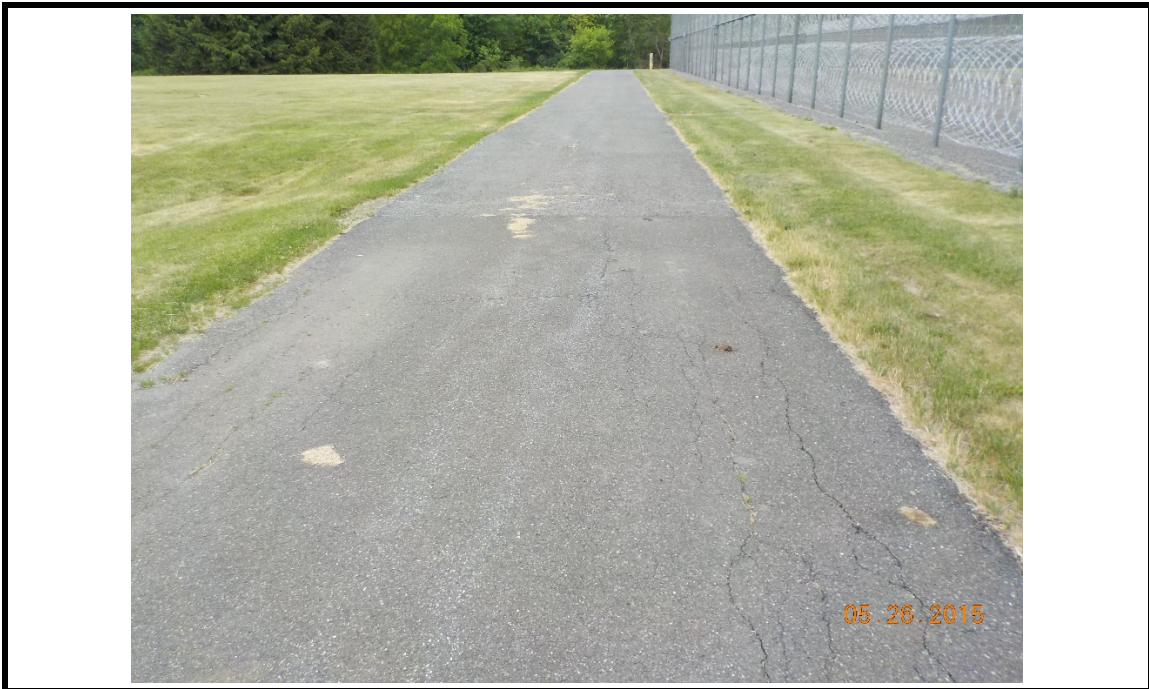
Photograph #2 - Description: Observed “Alligator” cracking at northeastern portion of patrol road. Looking east near B-2.
