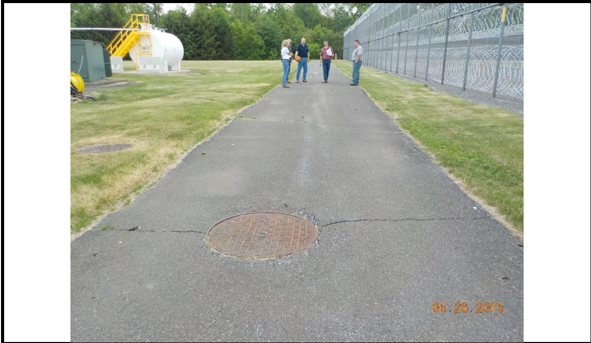
Photograph #1 - Description: Observed asphalt “block” cracking at northeastern portion of patrol road. Looking east near B-3.
