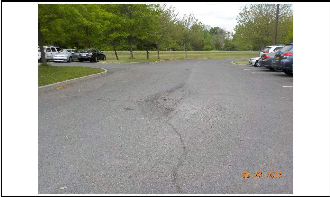
Photograph #3 - Description: Observed “Alligator” cracking along vehicle path. Looking west at entrance road.
