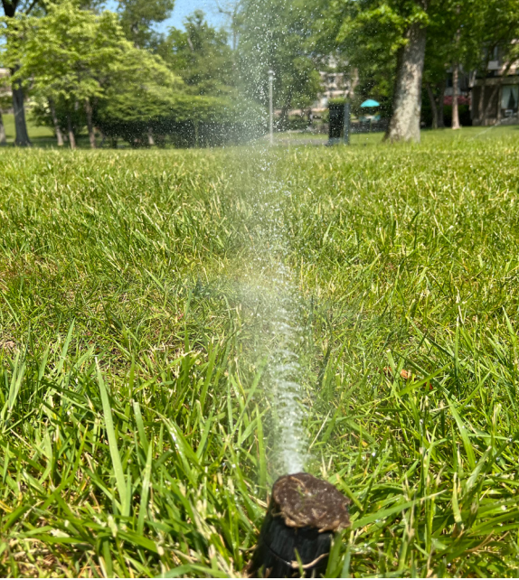
Stony Brook University (SUNY) installed 75 smart irrigation controllers to reduce water usage. Credit: Stony Brook University (SUNY)
