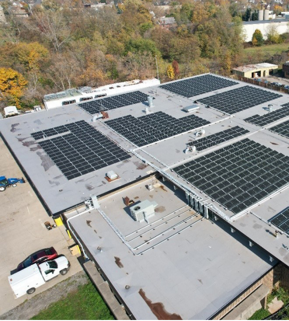
Parks Installed a solar array on a maintenance facility in Niagara Falls. Credits: Paul Vargovich, Jr. – National Solar Technologies and Parks
